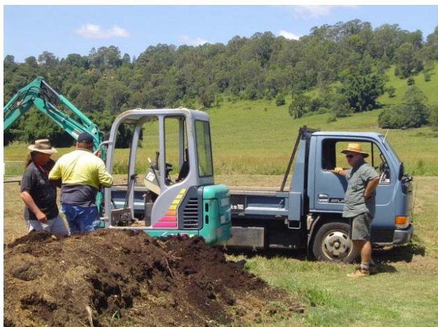
The first pile to go was the soil at the end of the shed, now helping to level the runway.
